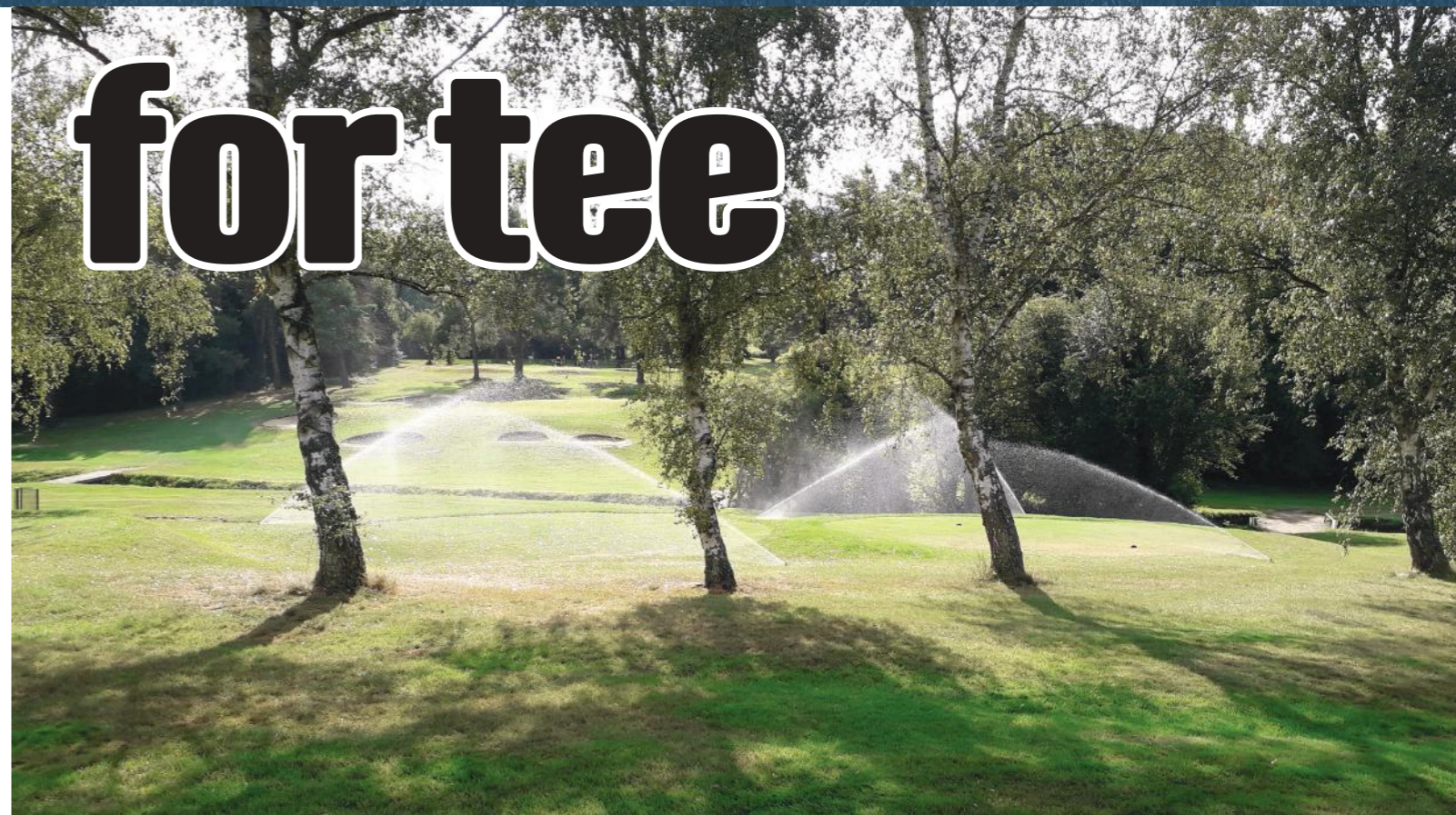
Rain Bird 5004 sprinklers on golf tee
